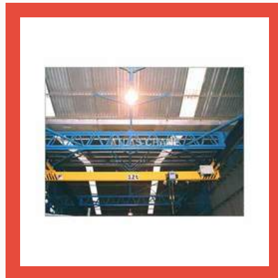
Underslung EOT Crane
